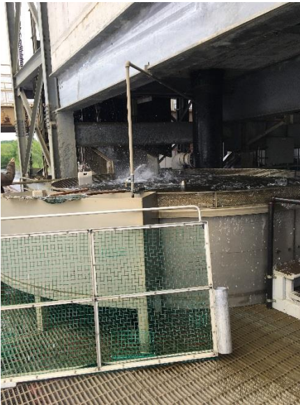
Trapping facilities at the Holyoke Fishlift. You can see a sloped flume underneath the concrete beam and a shad splashing into the holding tank. From here, shad are crowded through a pipe and into transport trucks.
